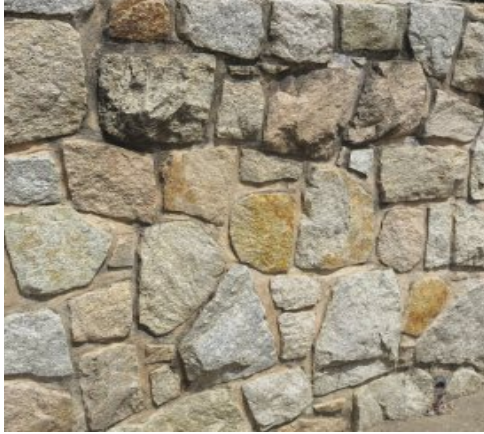
W1 Site stone retaining walls to match existing (seat height typically) retained or newly constructed
