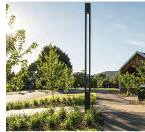
L2 Pole lighting to park - Supplier: BEGA Product Code: 77844
