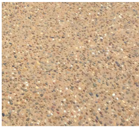
P1 Exposed aggregate insitu concrete (orange / sandy-coloured with rounded river pebble) with sawcut joints to match existing
