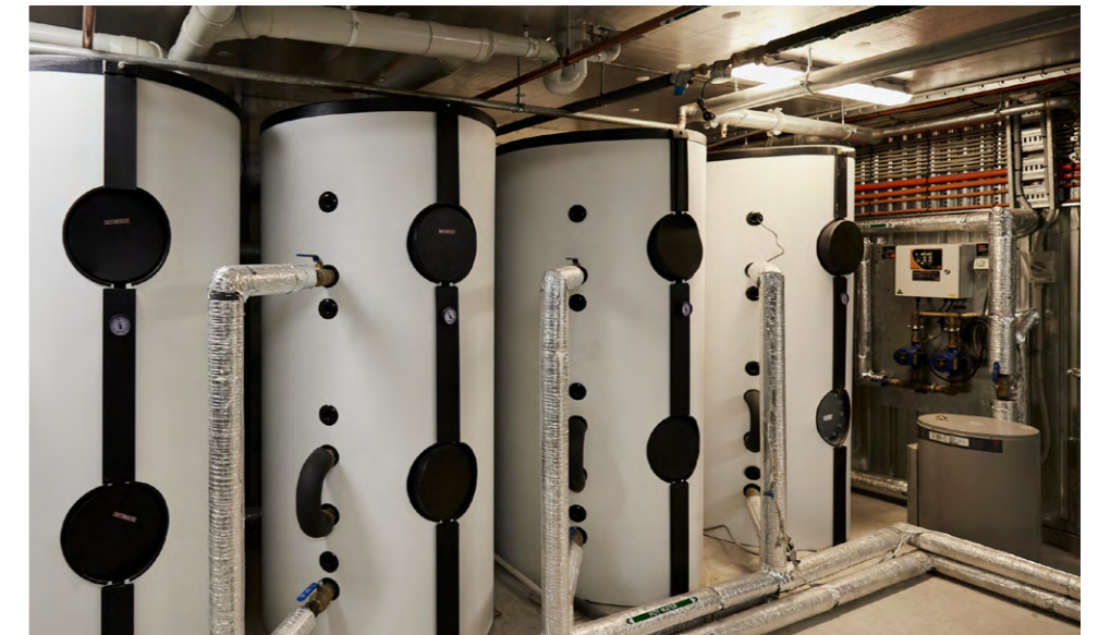
Heat pump systems. Image by Kim Landy.
